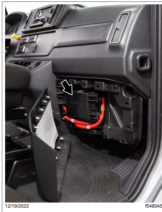
Fig. 8.7, Power Distribution Module (PDMi) Behind Right-Side Dash
